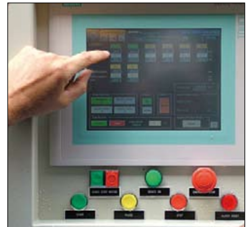
▲ PLC-controller station of the EPS-Series premium synchronous lifting system.
