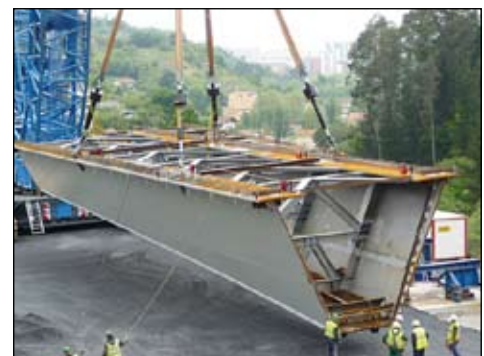
▼ Bridge segments are hoisted from the ground, being positioned with a 4-point SyncHoist system with fully monitorized cylinders.
