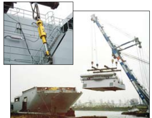
▲ Perfectly synchronised balance: Naval ship superstructure weighing over 600 tons placed on the hull using Enerpac's hydraulic SyncHoist.
